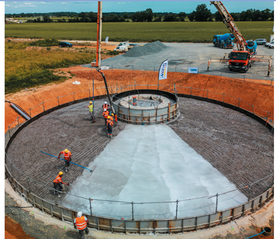
Plaine des Moulins wind farm in Jazeneuil (Vienne), pouring of a wind turbine foundation made exclusively of 0% clinker decarbonated concrete.
